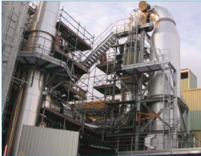
In this waste incinerator, AutoJet makes sure that the temperature of the combustion gases is lowered.
